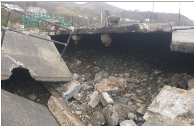
Figure 3. Storm damage in March 2020
