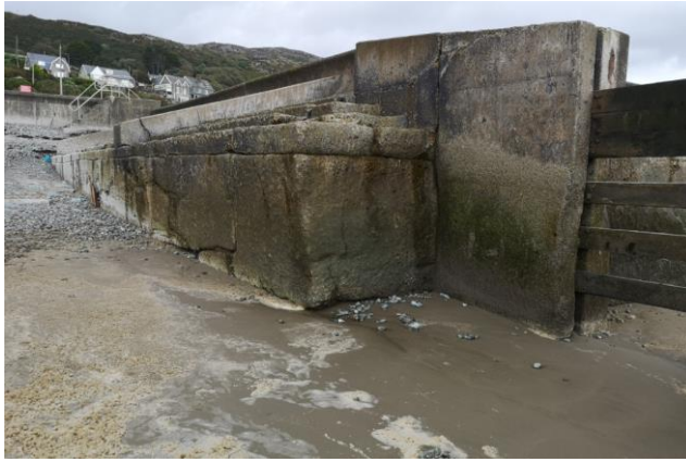
Figure 18. North-most end of promenade – concrete mass subject to significant deterioration
