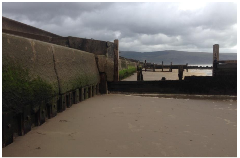
Figure 21. Groynes in very poor condition with limited impact on beach material movement
