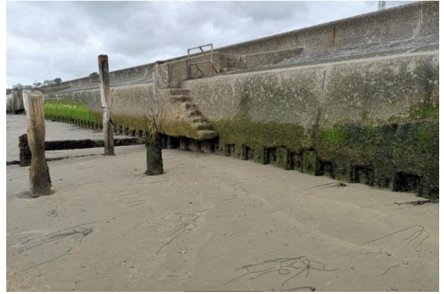
Figure 19. Northern extents of promenade – exposed sheet pile, with signs of draw down
