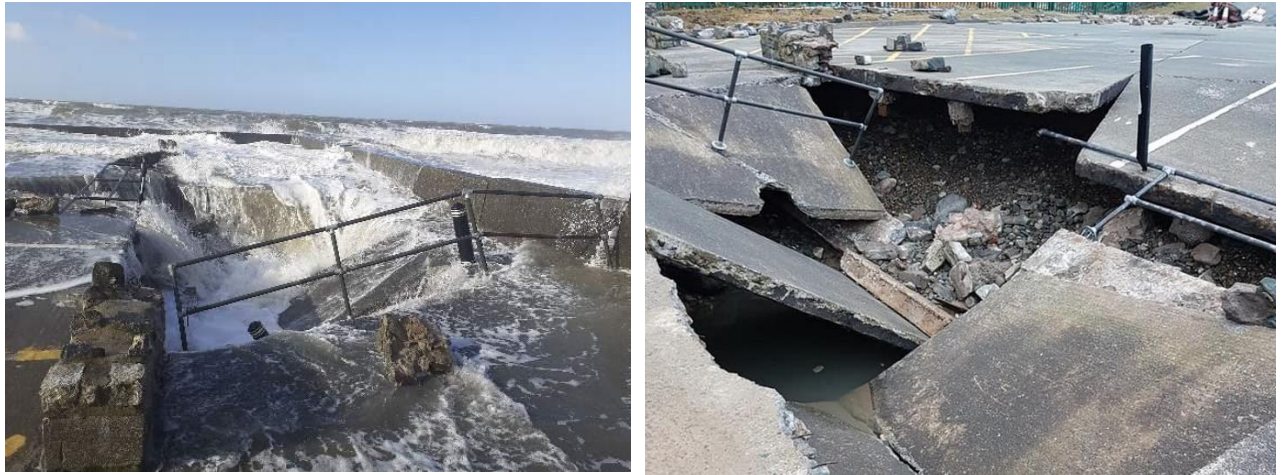
Figure 22. Damage to sea defences and collapse of the promenade at the north corner and return of Barmouth North Promenade in March 2020.
