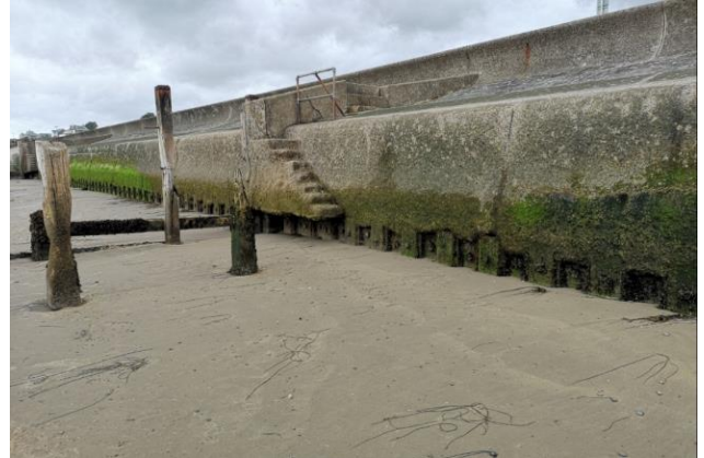
Figure 2. Northern extents of promenade – exposed sheet pile, with beach drawdown
