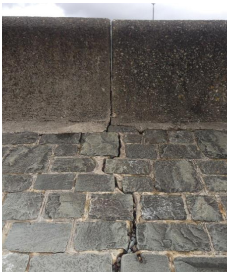
Figure 20. Promenade subject to cracking – notable void present at north-most end of the promenade.
